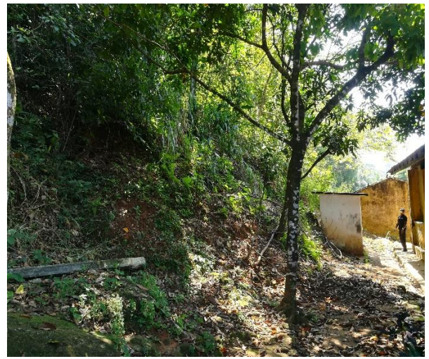
Figure 04 (d) – Slope failure impact the school building.
