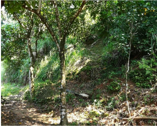
Figure 04 (a) – Failed slope as the result of no drainage available to discharge rain water.
